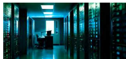
IN SERVER CENTERS
